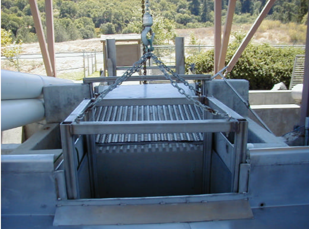
Figure 1-8 Adult Holding and Transfer Facilities at CVFF.
