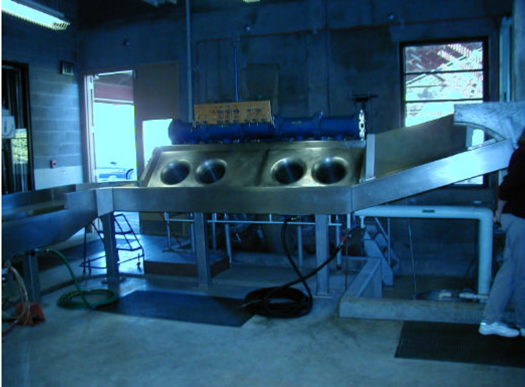
Figure 1-6 Adult Holding and Transfer Facilities at DCFH.
