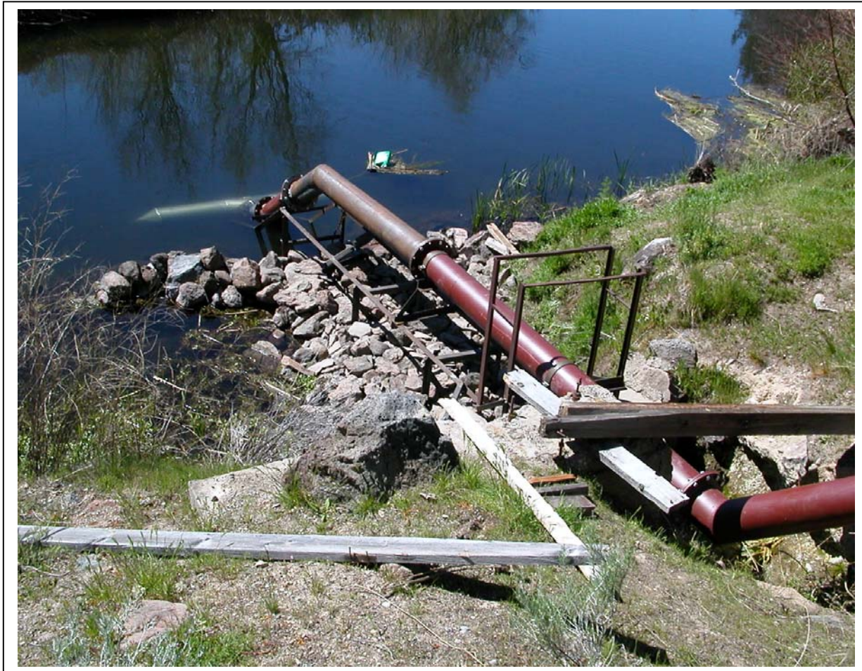
Final installation of the Nelson screen, at the beginning of the 2003 irrigation season.
