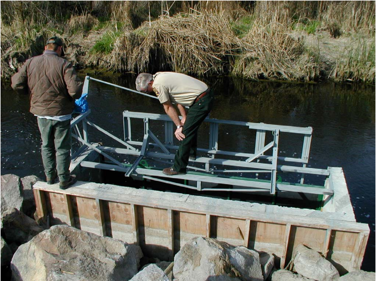
Mike Farmer and Ron Dotson (CDFG) inspect Fiock fish screen prior to installing covers and final backfilling.
