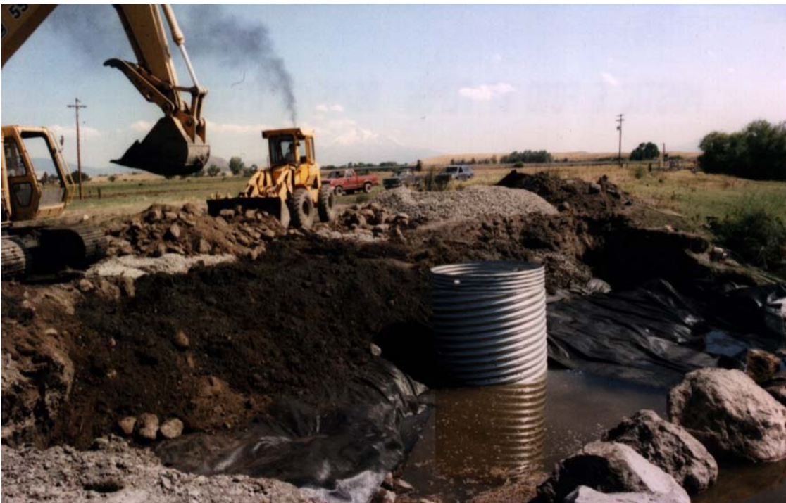
Replacing soil over infiltration gallery. Geotextile fabric in place to minimize movement of fines downwards into gravel.
