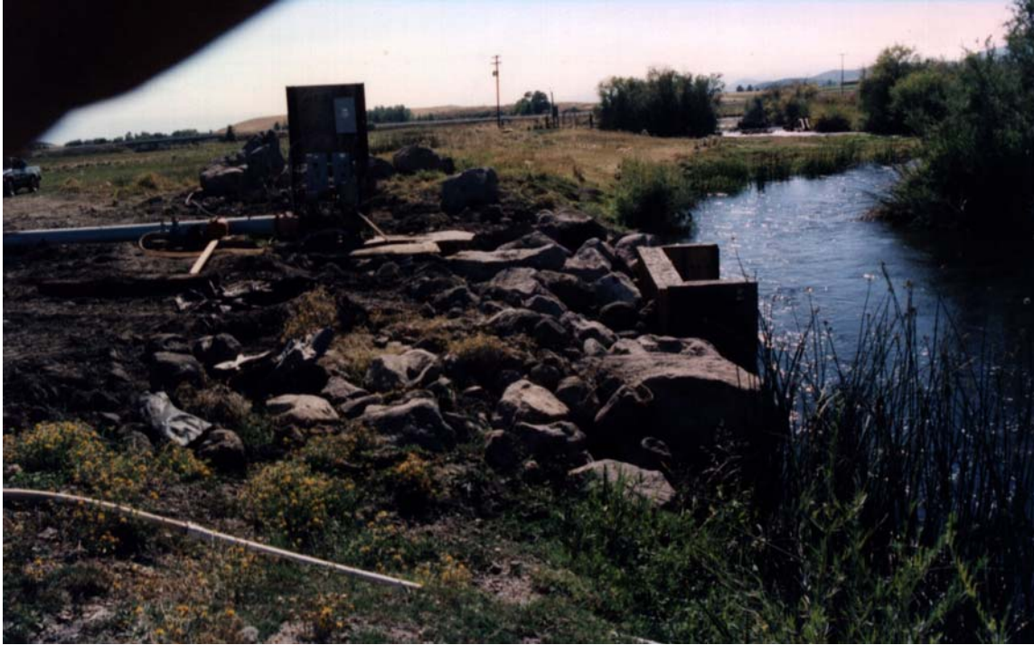
Concrete vault in place at end of irrigation season, 1999. Fish screen to be fabricated and installed over the winter.
