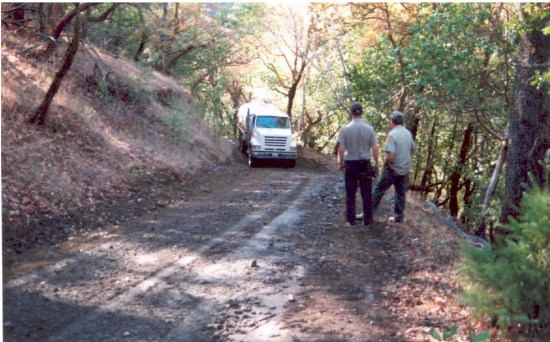
Figure 9. One hundred and thirty-six rolling dips were installed along roads in the Austin Creek State Recreation Area. Where appropriate, the road bed was outsloped, berms were removed and used to fill the inboard ditch, and broad, very driveable rolling dips were installed in order to disperse road runoff to the maximum degree possible.
