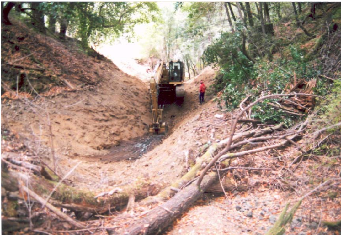
Figure 3A (top) and 3B (bottom). View downstream. Before and during excavation of channel stored sediment above undersized culvert stream crossing at Site #73. The culvert installation was a barrier to upstream fish migration and had also resulted in channel aggradation for 100 feet upstream of the culvert inlet. The stream crossing was properly closed by excavating all road fill and channel stored sediment upstream from the culvert.
