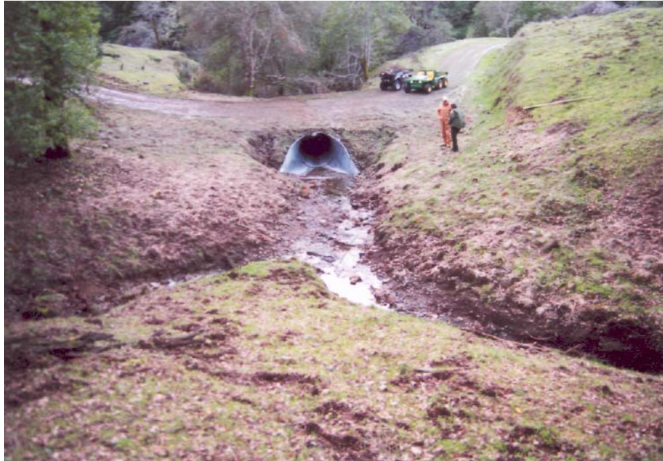
Figure 6. View downstream at Site #43 one winter after installation. Channel is flowing on bedrock with minor channel adjustments in cross sectional area, and the site has stable sideslopes.
