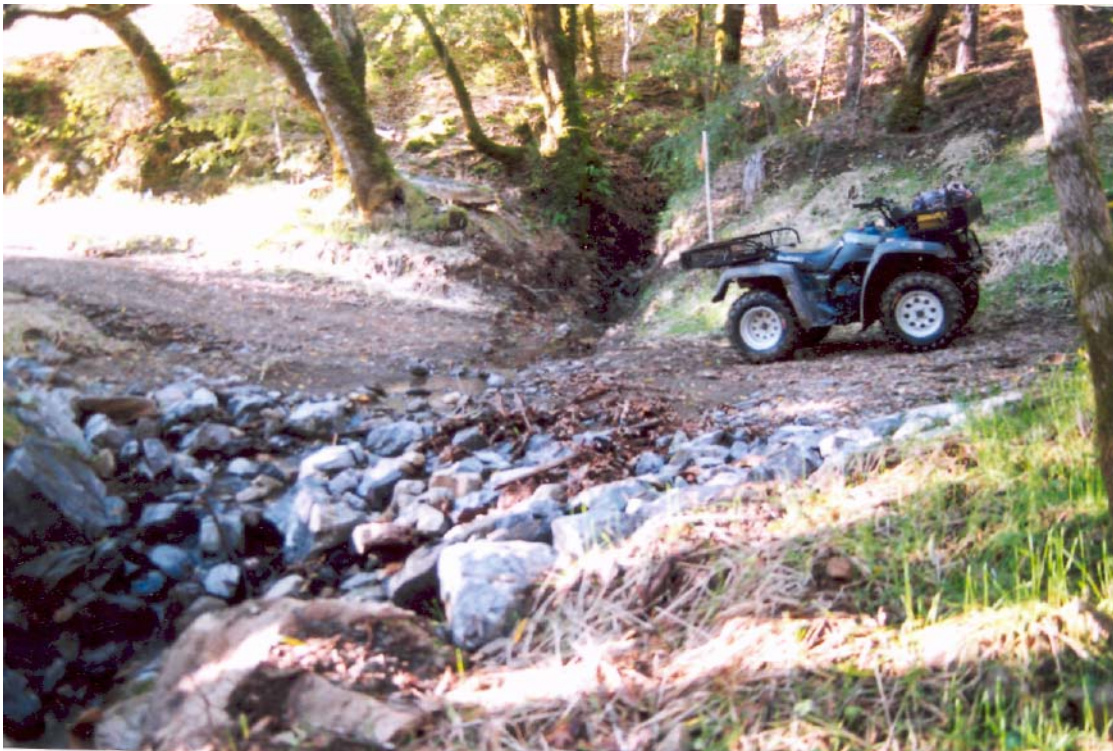
Figure 7. Twenty-three armored fill stream crossings were constructed in the East Austin Creek watershed during 2001. Armored fill crossings are appropriate along low use roads, and where properly sized culverts are difficult to install or where the culvert inlet would still have a high plug potential.
