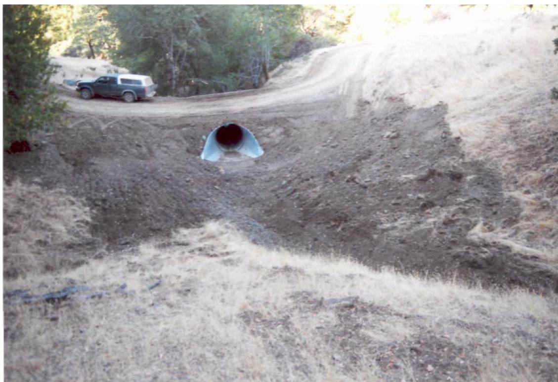
Figure 5 A (top) and 5B (bottom). View downstream at Site #43. Before and after photographs of upgraded stream crossing. Note prior and current culvert size, use of flared inlet to lower the plug potential at the inlet, use of low berm at outside edge of road to protect newly constructed fill slope and the excavation of channel stored sediment above the prior culvert inlet.
