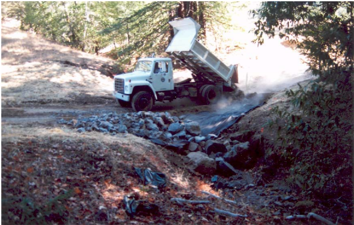
Figure 8A (top) and 8B (bottom). View upstream at Site #44. Before and during photographs of armored fill stream crossing installation. The shallow fill crossing limited the ability of Park Staff to install a properly sized culvert. Consequently, the culvert plugged frequently resulting in stream diversions and hillslope gullies. During installation, the road is lowered several feet vertically with a broad rolling dip, a keyway is dug from the base of the fill to the mid-point of the road bed, filter fabric is placed over the keyway, and a mix of rock armor is applied which is coarser than the stream is capable of transporting at high flows.
