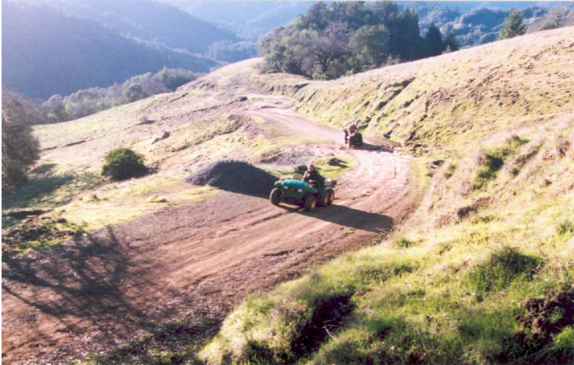
Figure 10. Often in grassland settings, ditches must be retained to insure a stable road bed. However, the road bed should be outsloped and berms removed, where possible, to disperse fine sediment originating from the road bed off the outside edge of the road, and not be delivered to live ditch. Heavy fall rains terminated the project last year prior to final road grading and the distribution of road rock. Some rilling of the road bed occurred during the winter. This section of road was recently re-graded to improve the outslope and insure the road drains properly in future years.
