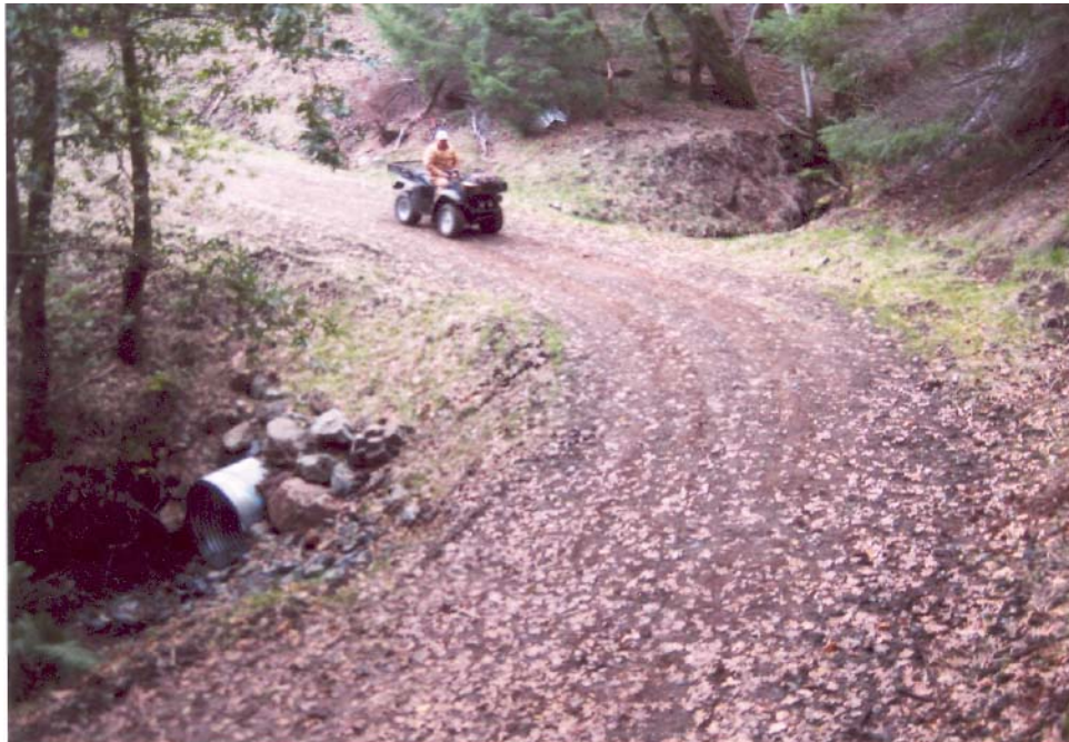
Figure 4A (top) and 4B (bottom). Thirty-one stream crossings had culverts installed which were sized for the 100 year storm. The culverts were installed at the base of the fill in line with the natural channel, had sufficient culvert length to construct stable fill slopes and were fitted with critical dips to prevent future stream diversions.
