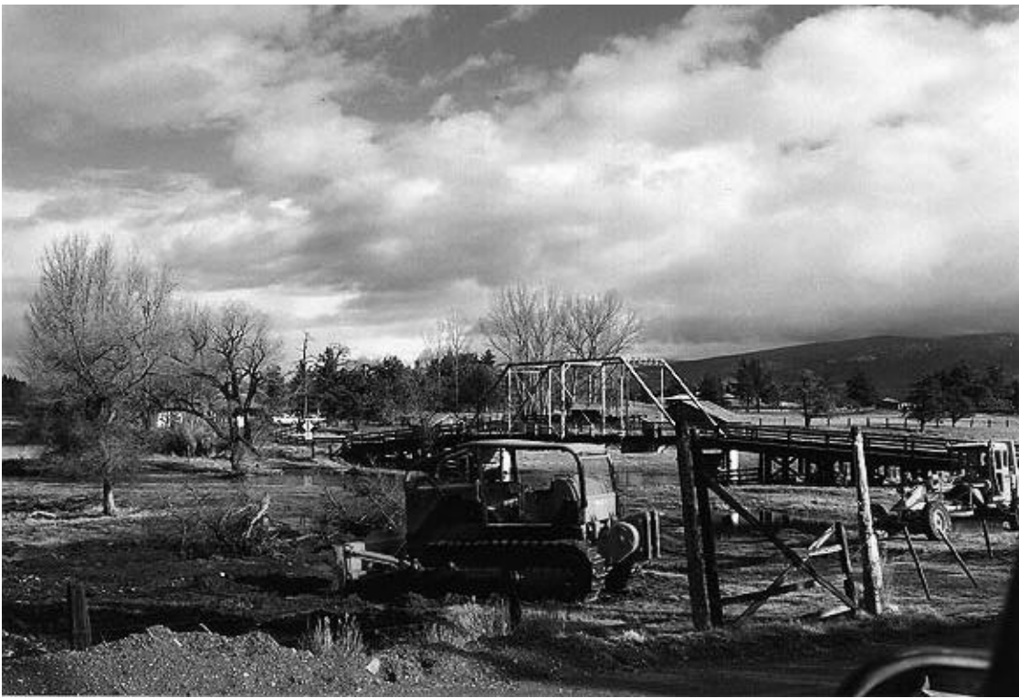
Figure A5-45. Riparian zone of the Shasta River at Louie Road with heavy equipment and filled riparian wetlands.
